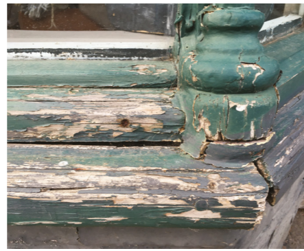
Timber bay modern paint failure on Listed Building.
