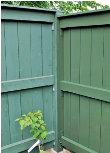
First and second coat. FINISH PAINTING! At least three fully covering coats.
